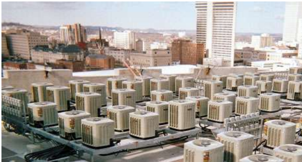
Photo for illustration purposes - area between units open for air to draw from top, bottom, and sides.
