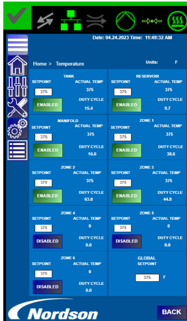
Figure 5-5: Temperature controls setup screen
